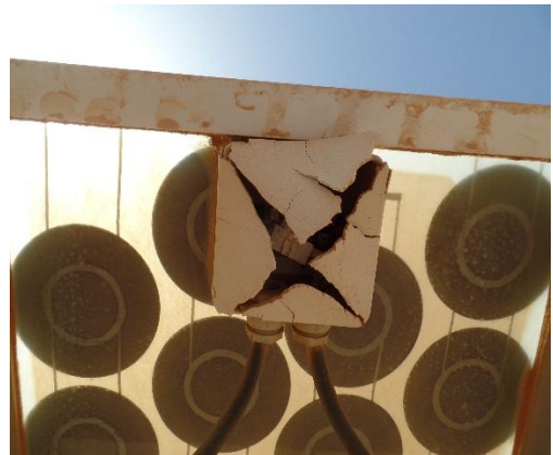
Fig.9. Junction box damage (back side of PV module)
