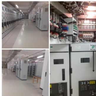
A.7: Electrical control room
