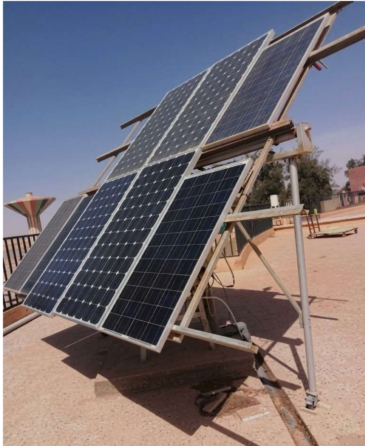
Figure III.8: SOLO LINE LX-100M photovoltaic panel installed at URAER [33].
