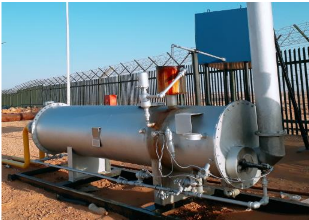
Figure III.12. Chauffage de gaz lift.
