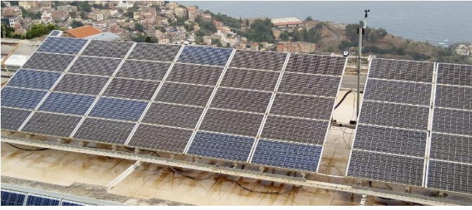
Fig 1. Picture of PV Array of the GCPV system on the administration roof at CDER
