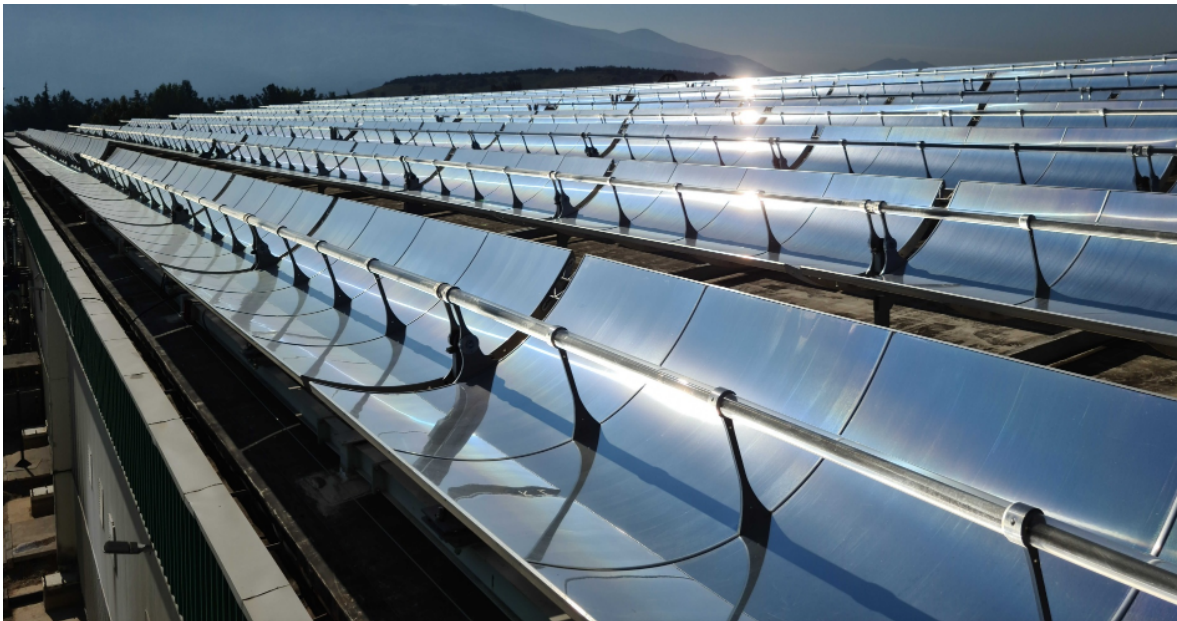
Figure I.7: Parabolic trough collectors
