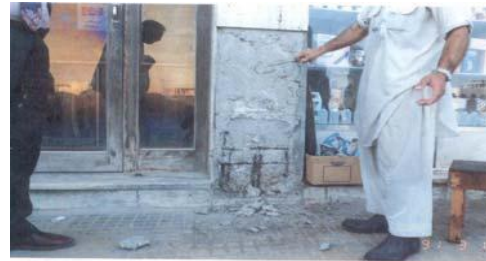
Corroded Re-inforcement in Column at the front
