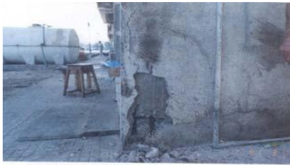
Corroded reinforcement in the Ground Floor Column at the corner
