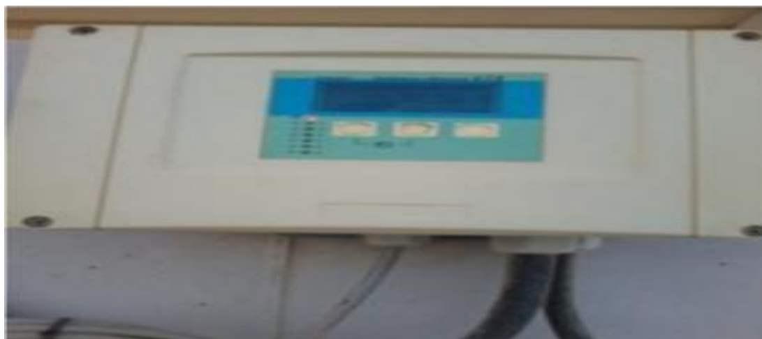
Figure 06: Image of the inlet and outlet water meter (Débit meter) (ONA,2023).
