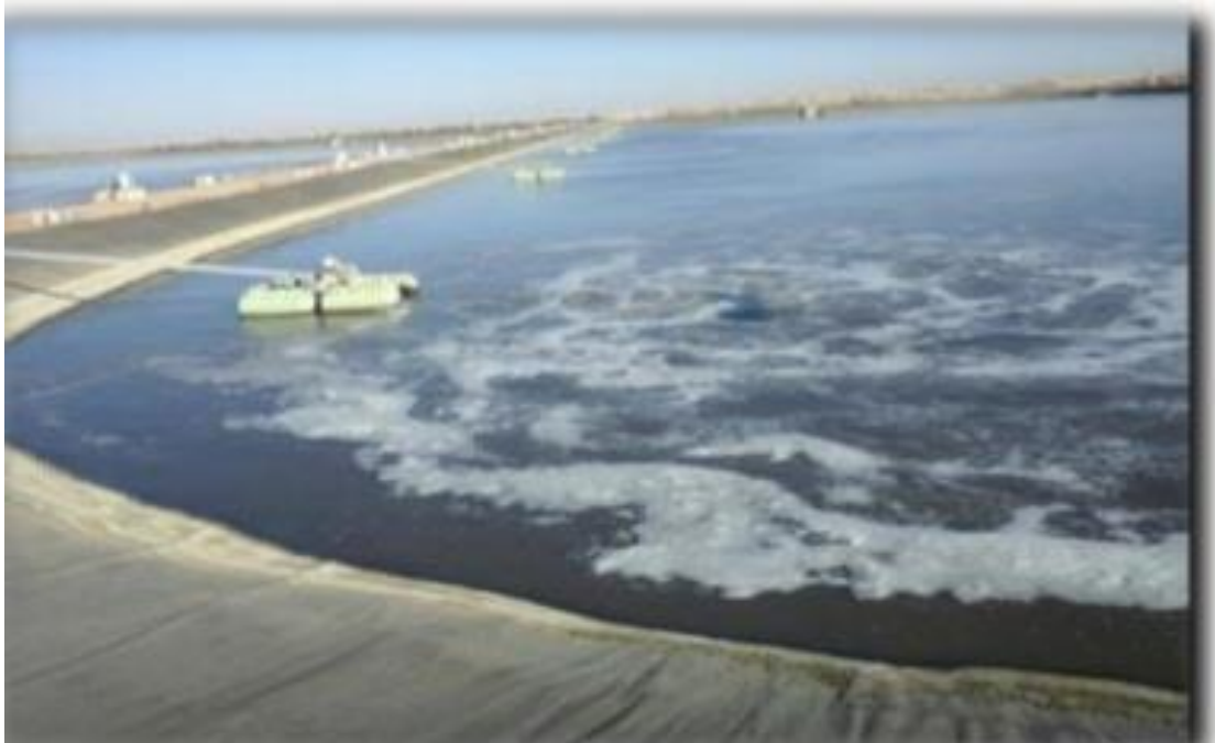
Figure 12: Aerated basins in the first stage (A1.A2.A3). (ONA,2023).
