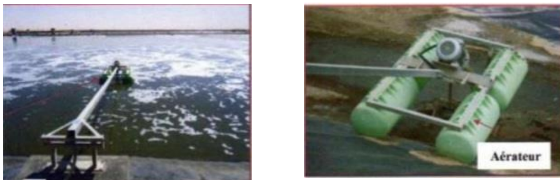
Figure 14: Aeration pumps inside the basins (ONA,2023).
