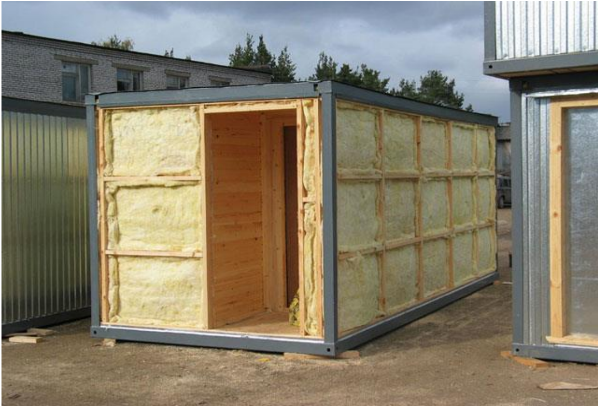
Figure I.12. Use of mineral wool to insulate the exterior walls of the house
