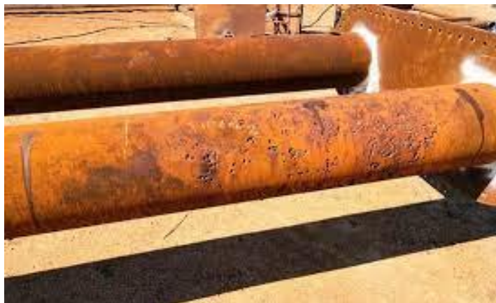
Fig.I.11: forme de corrosion.
