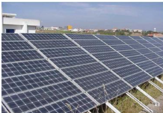
Figure I.29 Champ photovoltaïque fixe [12].
