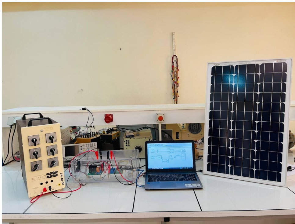
Figure VI.19 :Real photo of PV system.
