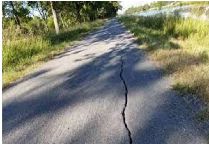
Figure 2.7: Fissures de rives
