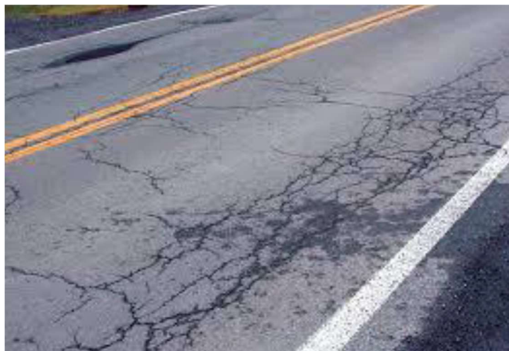
Figure 2.8: Fissures de gel
