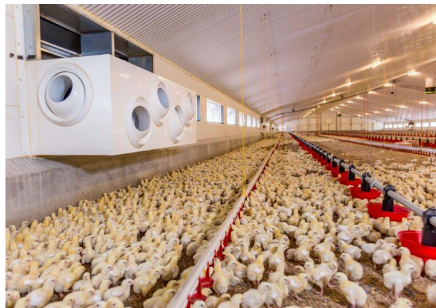
Figure 14 : Air installation in poultry houses [39].
