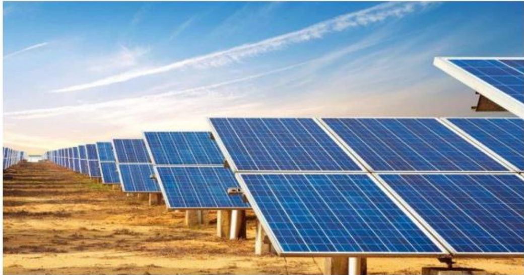
Fig.2.1. Fixed photovoltaic field [4].
