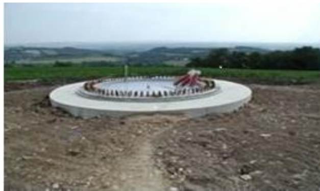
Figure I.8: Wind turbine basis.
