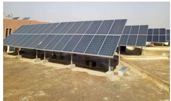
Fig. 1. View of the PV plant installed in the roof of URER-MS, Adrar.
