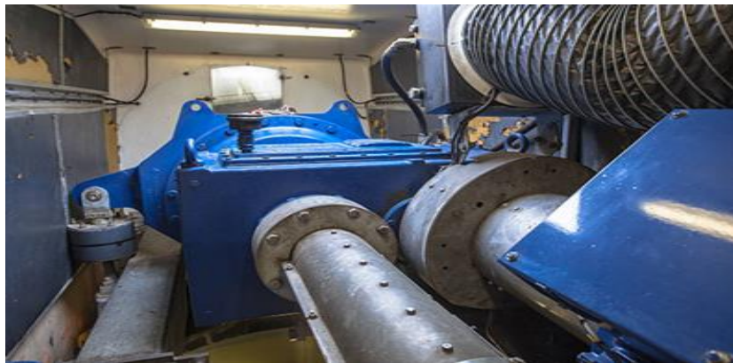
Figure I. 4 Inside mechanical components of the nacelle
